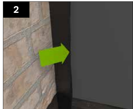
At the host wall fold the vertical DPC over the top of the membrane prior to battening out.
